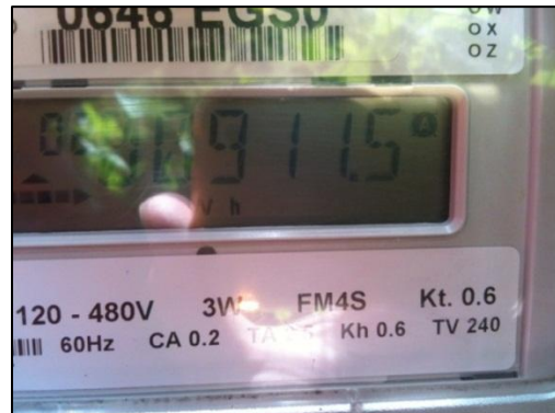
Final meter reading @ 1200 hrs on 16 July 2012
