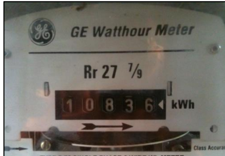
Initial meter reading at 1600 hrs on 20 Feb 2012
